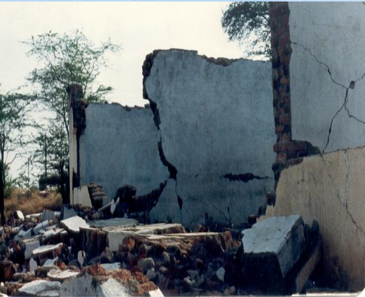
Plate 1: Out-of plane collapse of wall of a school building (Sastur)
