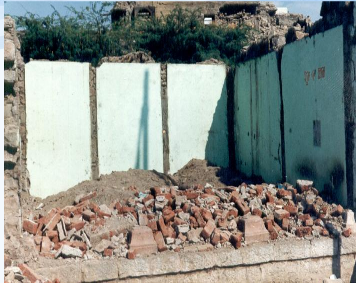
Plate 2: Timber post supported wall of a shop building intact after earthquake (Sastur)
