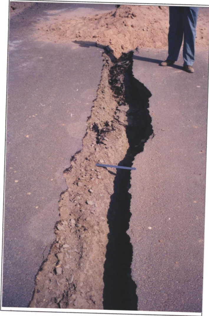
Road Embankment failure
