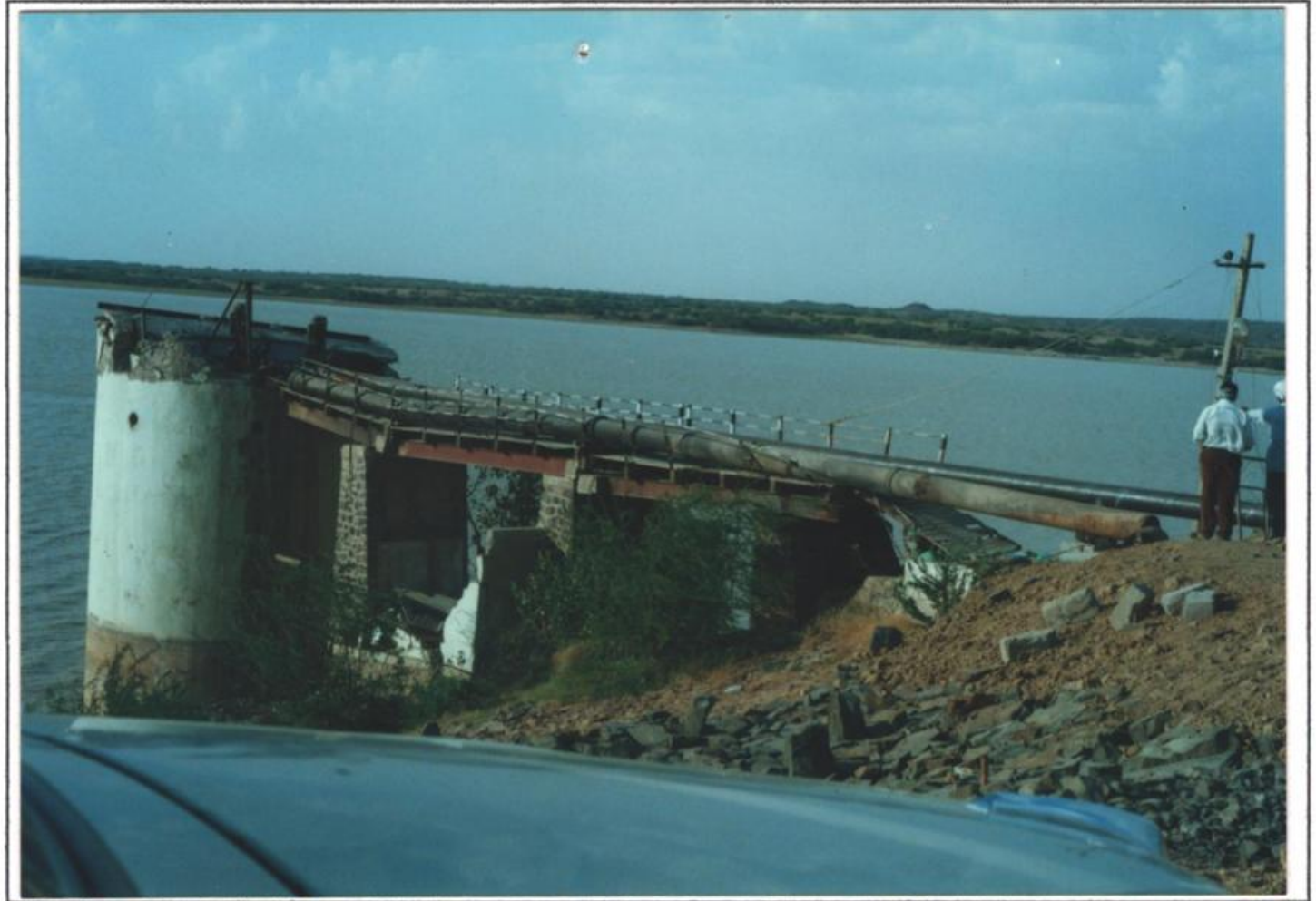
Collapse of the Intake Structure at the Tapar dam
